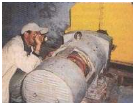
NUNV DN Adhikari observes the broken fan in the generator
