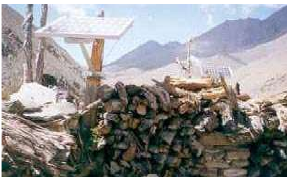
An RADC Solar panel installed in Dho, Dolpa District
